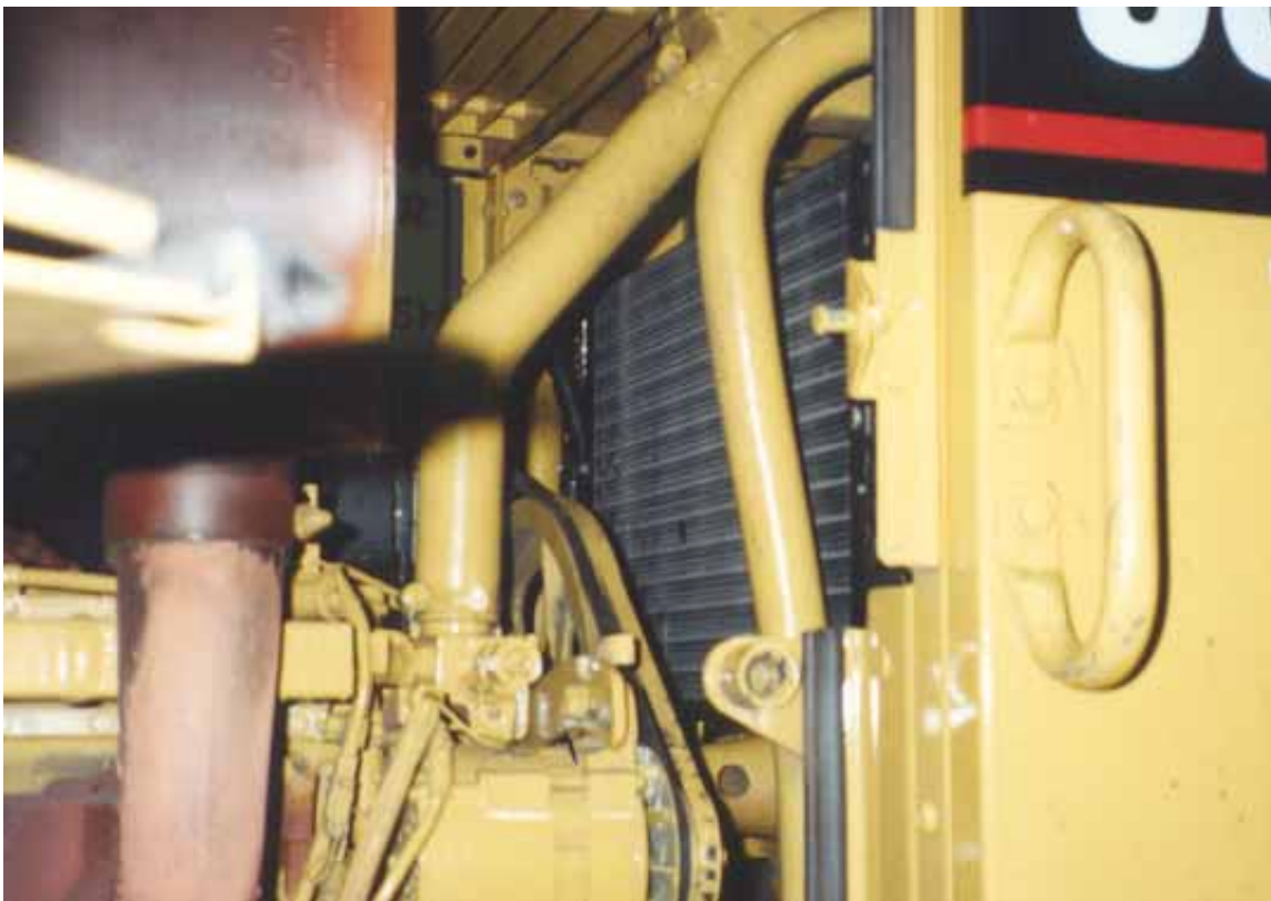
Condenser as viewed from left side.
