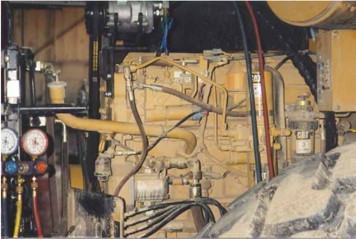
Compressor in place showing line runs.
